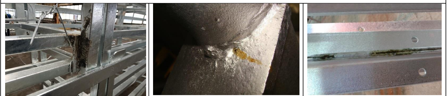
Untight welds – blow-outs and leaks are not sealed
